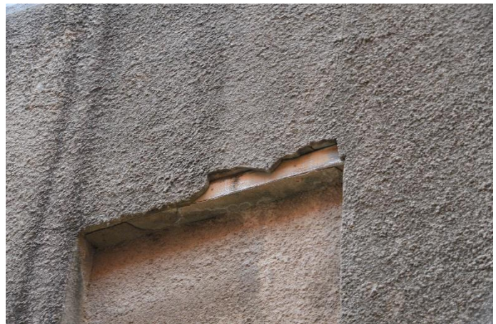
Exterior damage in same area
