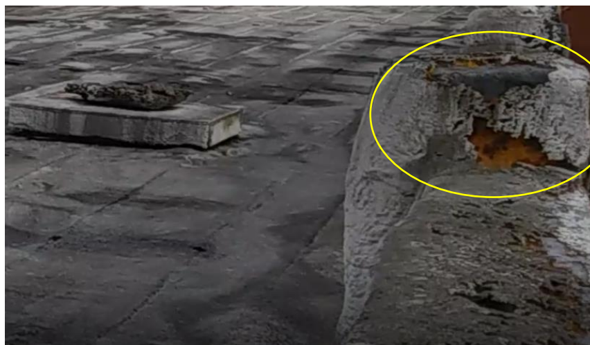
Damage along parapet
